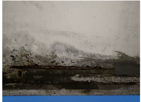
Photo 4 - Spalled concrete delamination with exposed reinforcing bar and metal connector.
