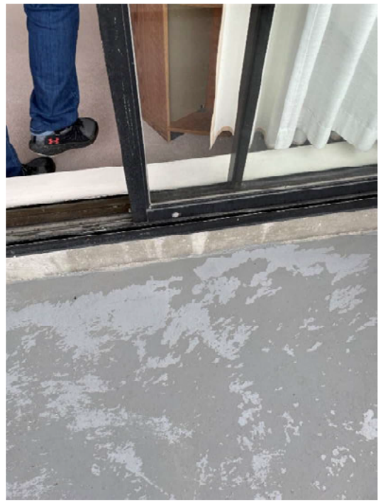
Photo 18 - Peeling paint on balcony floor.
