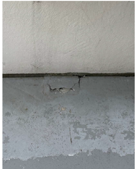
Photo 3 - Spalling concrete above pre-cast panel connection to the balcony slab.
