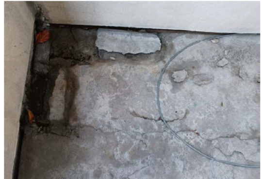
Photo 2 - Concrete delamination on balcony - slab.
