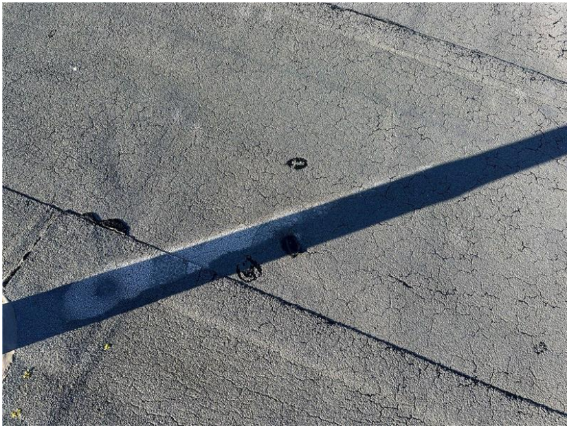
More damaged membrane.
