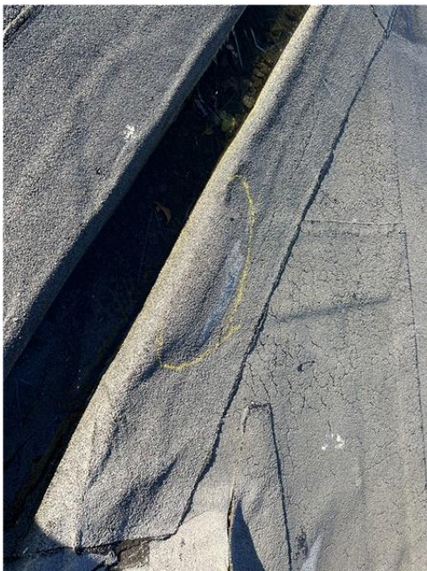
More damaged, wrinkled and blistered membrane.
