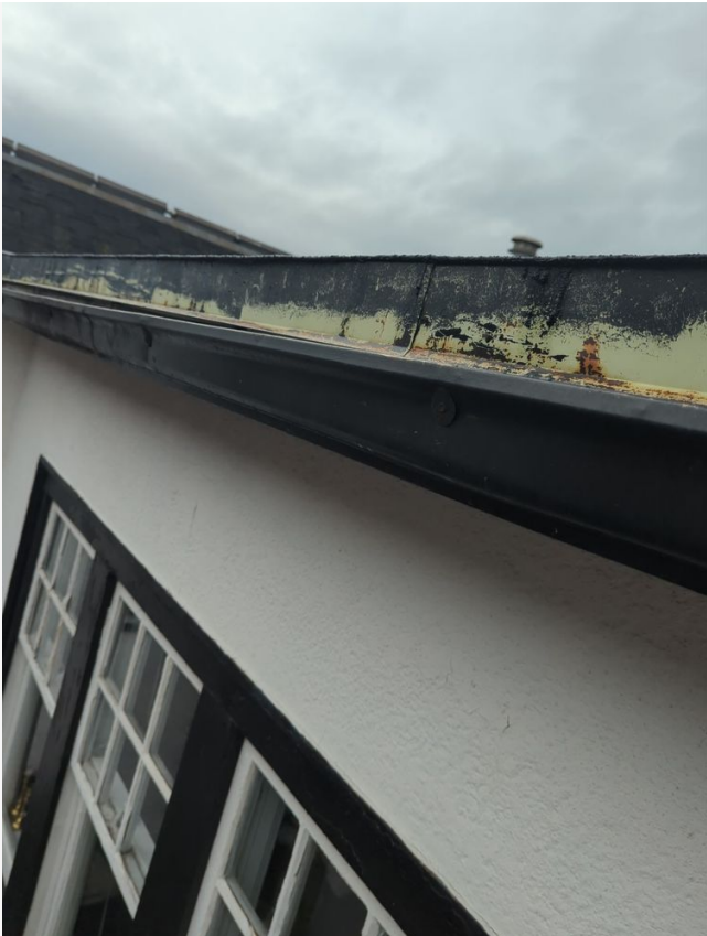
We will replace this rusty flashing system.
