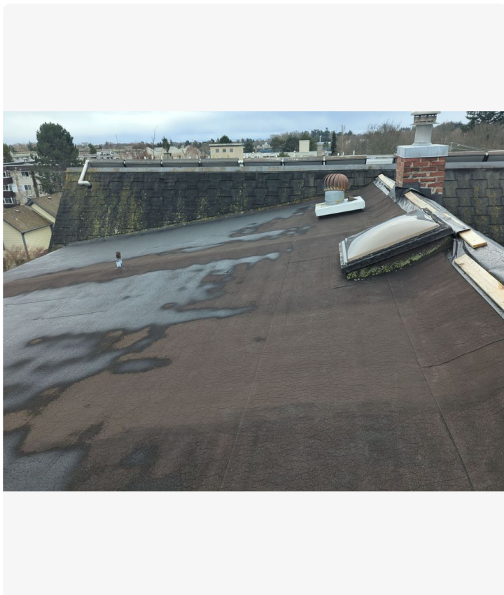
The flat roof is ready for replacement. I have quoted it based on a 1 layer tear off. We will need to take a core sample to confirm if this is accurate.
