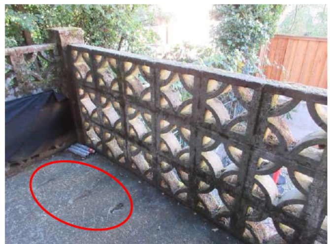
Photo 4: Typical 1 st floor balcony/patio guard; note three locations of exposed reinforcing steel within the red oval.
