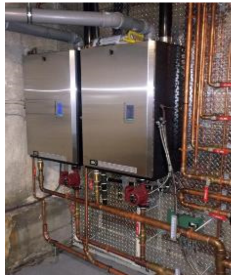
Example of upgraded condensing boilers
