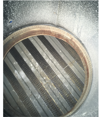
Image of the heat exchanger from within the flue stack; corrosion evident, likely from condensation.
