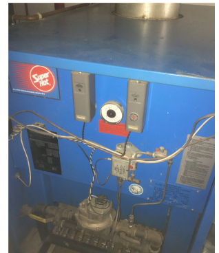
Existing SH boiler
