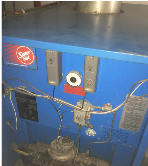
Existing space heat boiler; low efficiency
