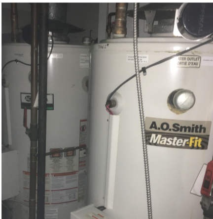
Existing DHW tank heaters
