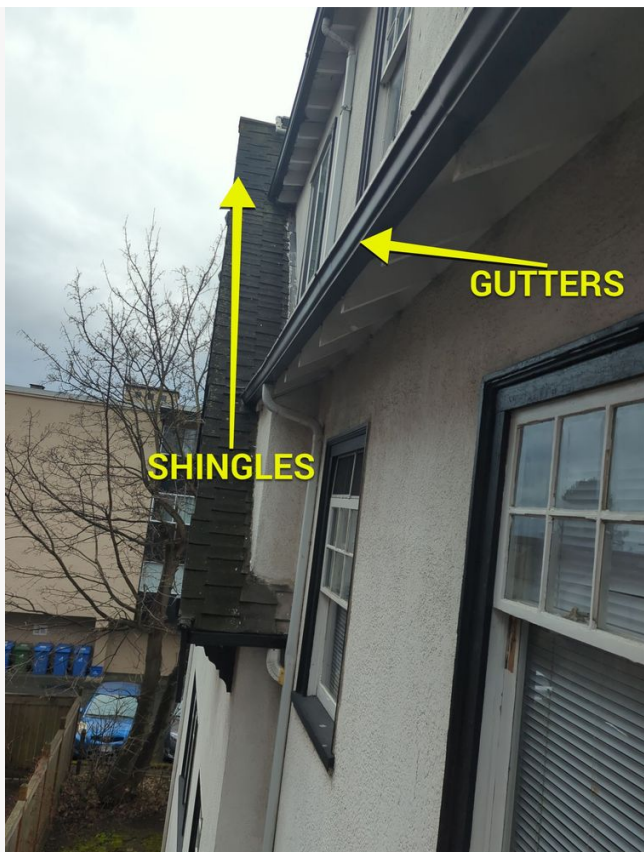
The gutters and downspouts were well passed the end of their service life. The shingles were also well passed their service life.
