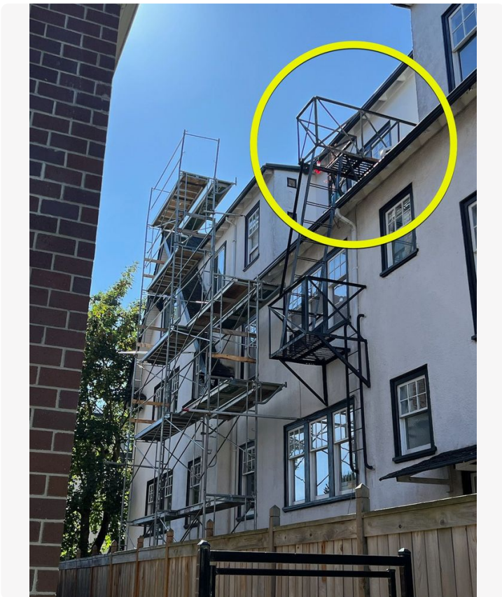
This fire escape needed a lot of work to keep it functional for the long term.
