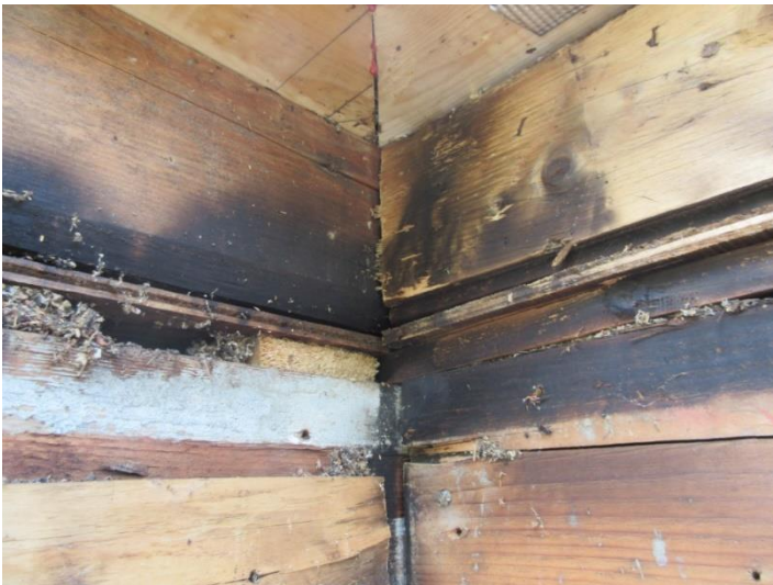
Photo 3): Burn marks at framing on the north elevation.
