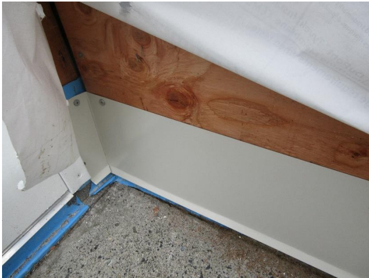
Photo 3): Self-adhered membrane not fully extended behind base of wall flashing.
