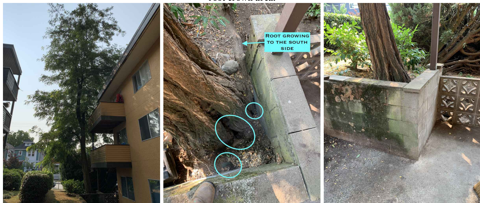
Tree #37 – North and west rooting area restricted by a retaining wall. Gaps can be found at the root crown area.
