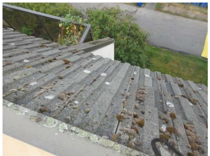
Photo 15: Typical mansard roof with vegetation growth.
