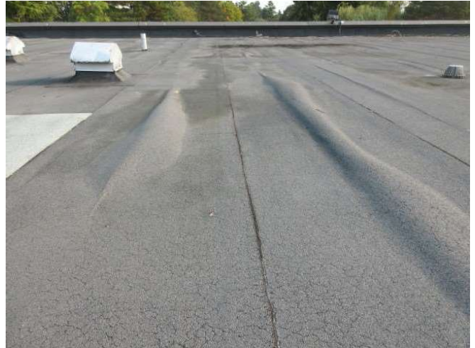
Photo 13: Typical older modified bitumen roofing with blisters, ridges and cracked waterproofing.
