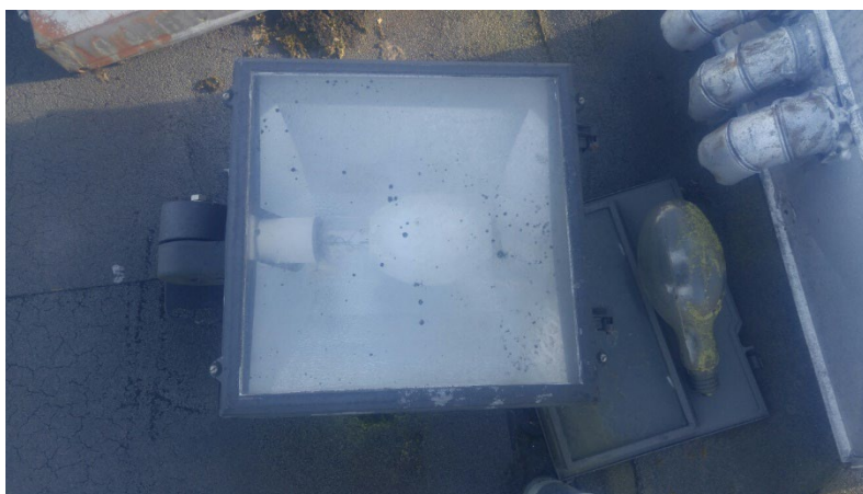
Photo 3 – Defunct HID bulbs on roof
