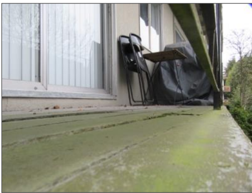
View of water staining and organic growth on the wood deck boards serving a balcony system.
