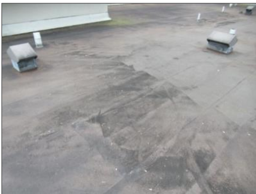
View of evidence of ponding water atop the north roof system.
