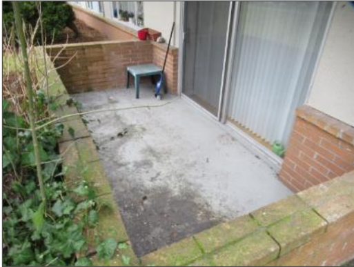
View of a grade level patio on the north elevation of the Site Building.
