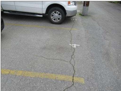
View of cracking in the asphalt paved parking lot.
